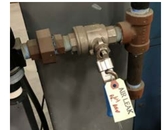
Identified and tagged air leak
