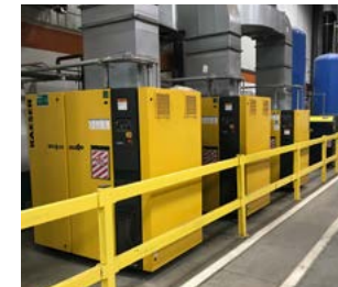
Compressed air system generators
