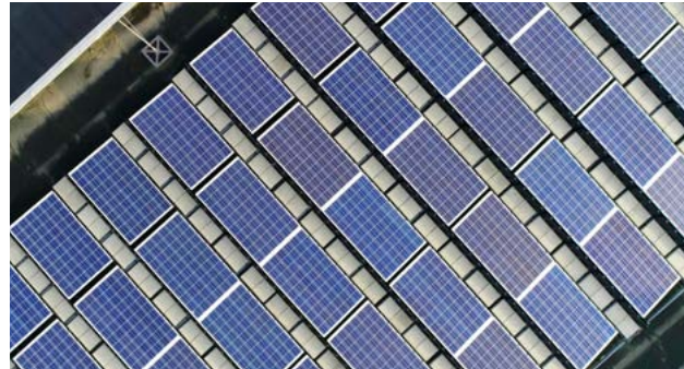
Solar panels installed on the technology rooftop have produced 26% of the total energy consumption, exceeding the planned target output.
